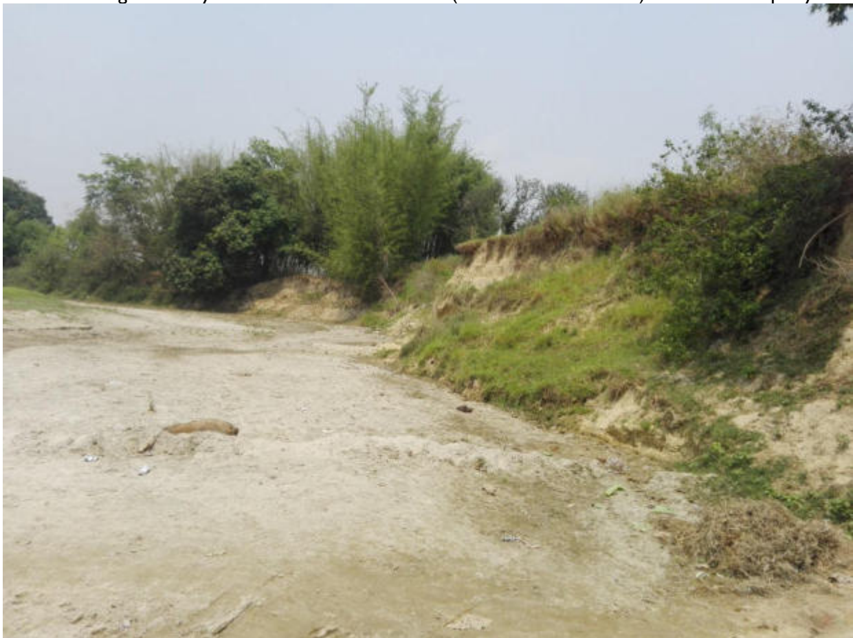
River banks cutting through agriculture lands needed stabilization (26.641745/86.593877) Khadak Municipality-5
